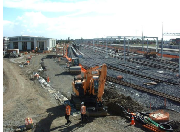
Fig 6: Installation of utilities and trackwork - note overhead line gantries in the background
