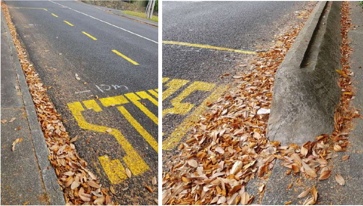
Figure 25: Accumulated debris near the bus stop blocking the channel.
