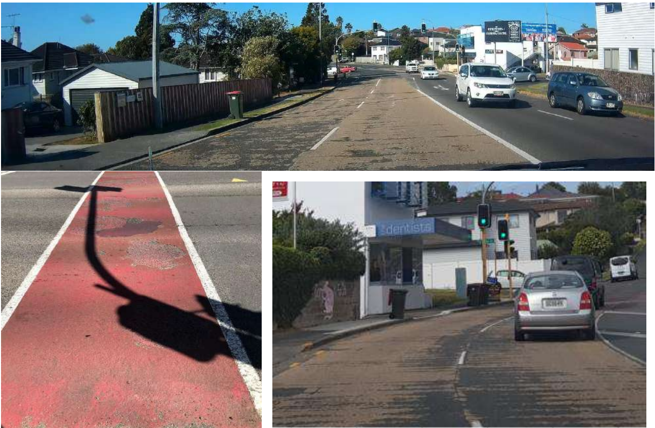
Figure 16: Poor conditions of the current high friction surfacing and red colour surface treatments between the pedestrian cross walk lines.
