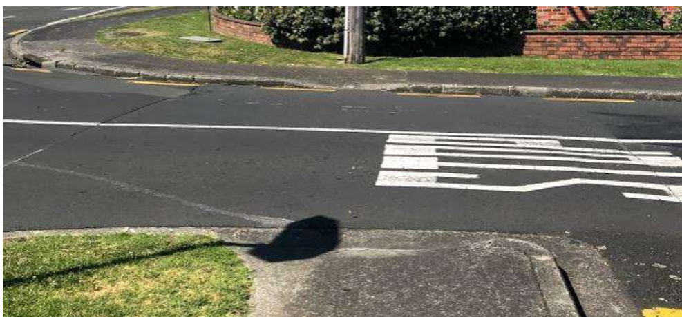
Figure 18: Substandard pram ramps at Littlejohn Street Intersection
