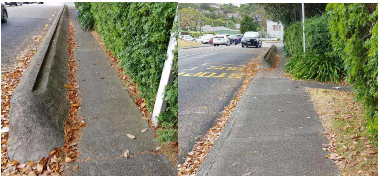
Figure 6: Concrete wall and vegetation reducing the usable width of the footpath near the westbound bus stop near Frederick Street.
