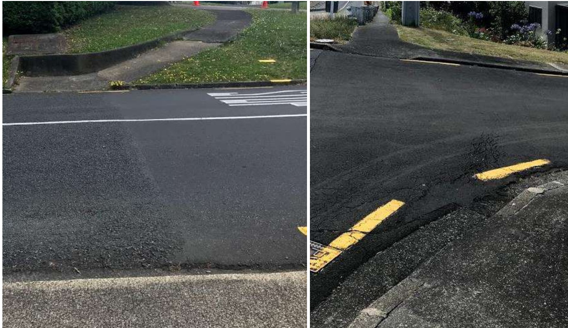
Figure 3: Pram crossing facilities in poor condition across Frederick Street and Lilac Grove.
