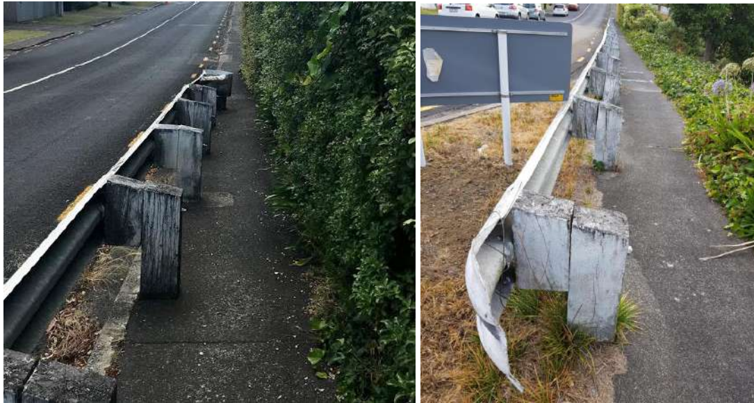
Figure 7: Existing barrier reducing the usable width of the footpath
