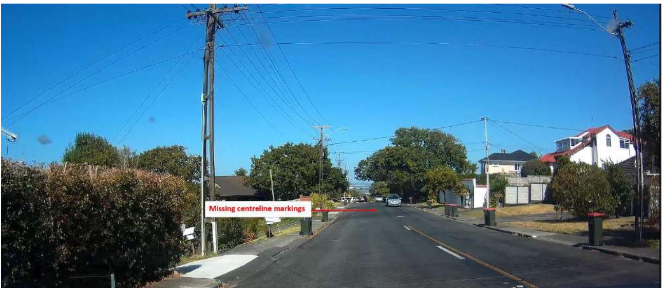
Figure 10: Missing centreline marking along the corridor
