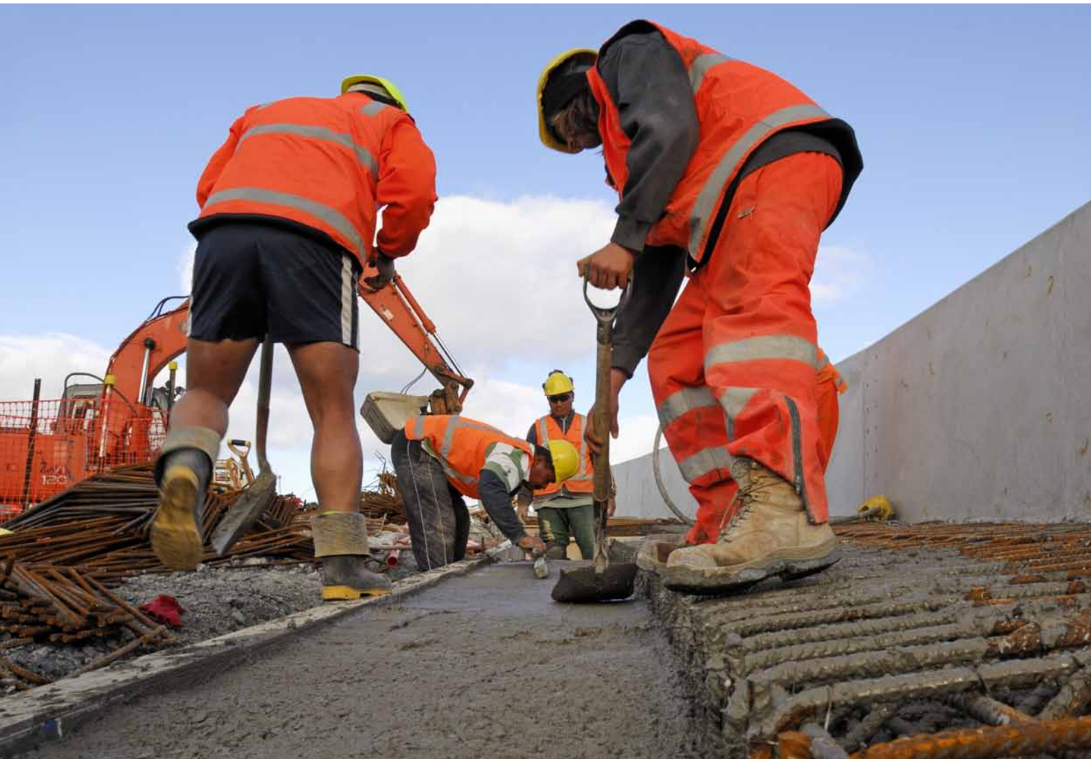
A new bridge over the rail trench in New Lynn will create a bypass of the town centre for heavy vehicles on SH20
